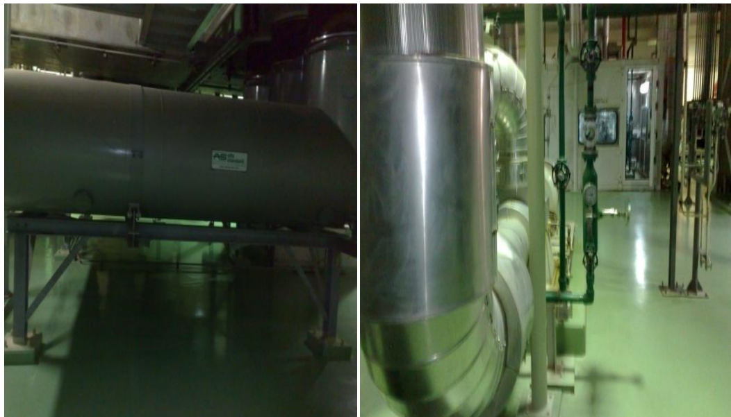
Figure 3.11 At generator,( STU3)
