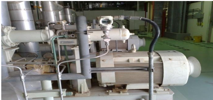
Figure 3.3 at low pressure feed pump,( STU3)
