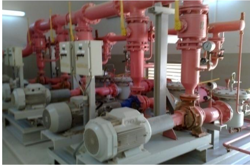
Figure 3.26 4,20 m from X23 inside room, (FFPU)
