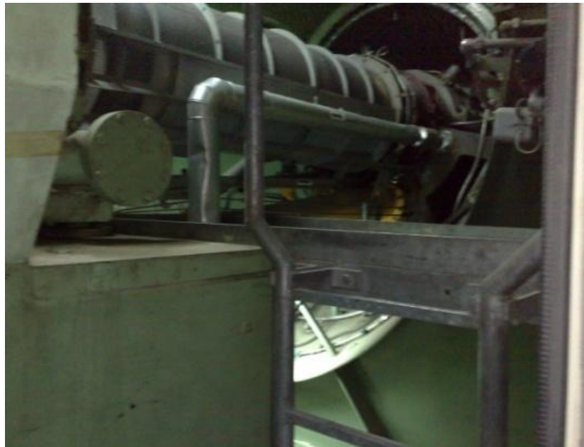
Figure 3.31 At the door (1) to trust bearing joint between compressor and generator room, (GT14)
