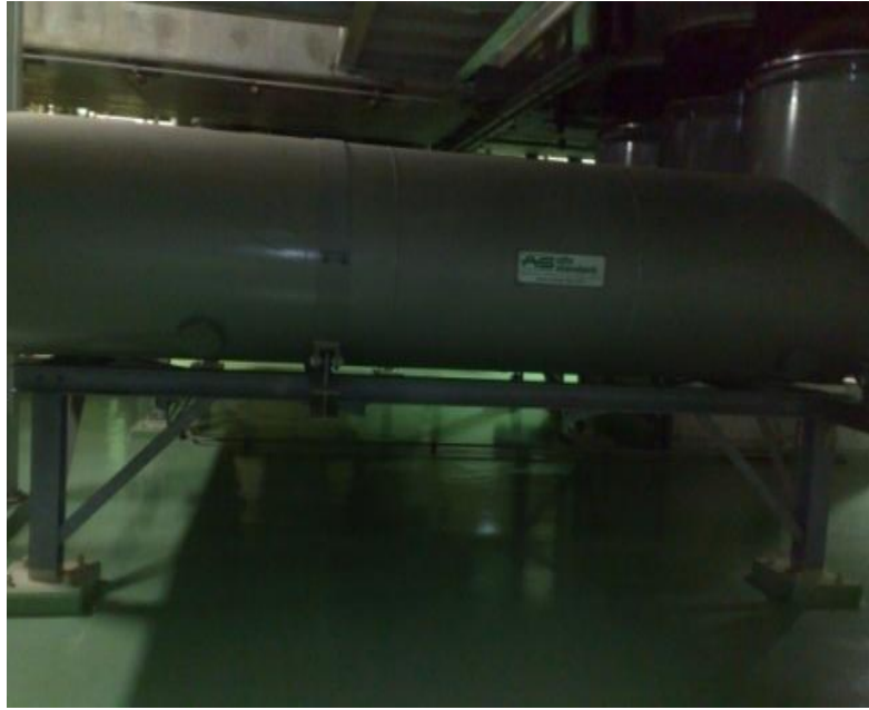
Figure 3.22 At generator, (STU1)
