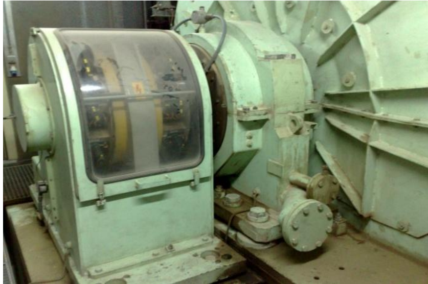
Figure 3.34 At the door generator room, (GT14)
