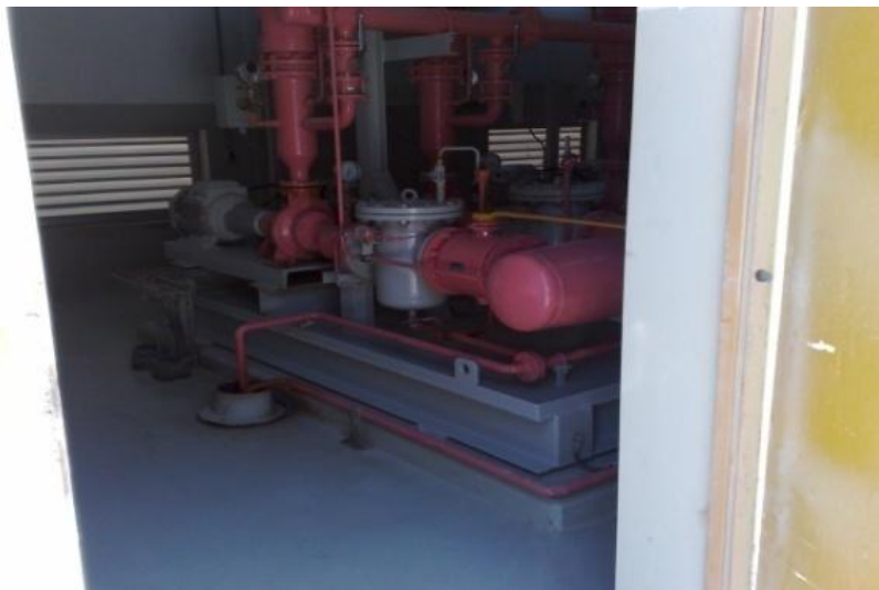
Figure 3.25 At the door fuel forwarding pump, (FFPU)
