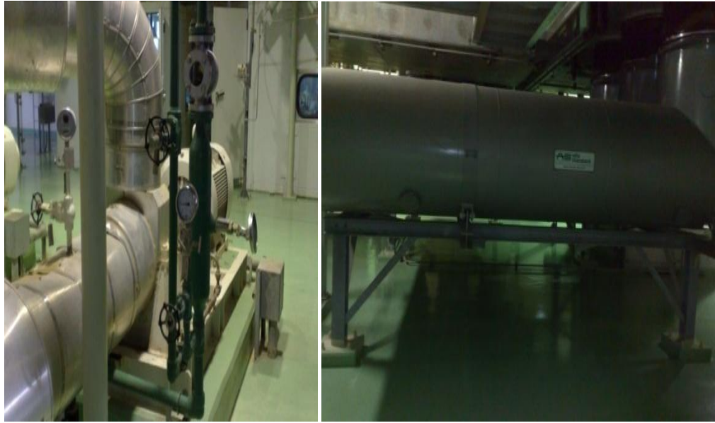
Figure 3.16 At generator,( STU2)
