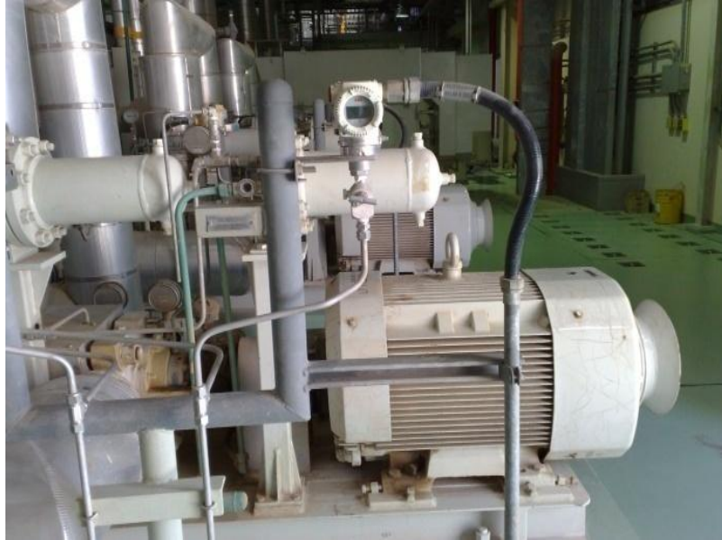
Figure 3.12 At low pressure feed water pump,( STU2)
