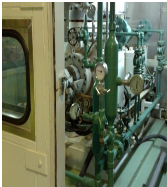
Figure 3.19 High pressure feed water pump, (STU1)
