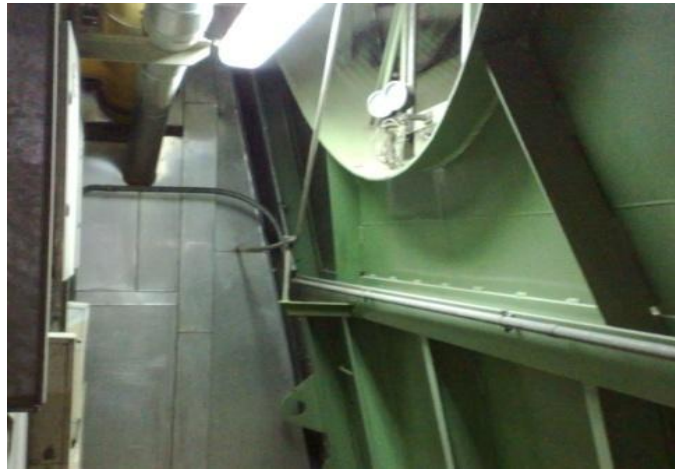
Figure3.32 At the door (2) to trust bearing joint between compressor and generator room, (GT14)
