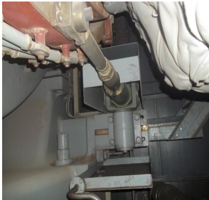
Figure 3.33 At the door gas turbine room, (GT14)
