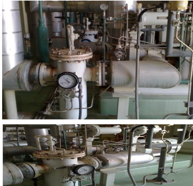
Figure 3.18 Low pressure feed water pump, (STU1)
