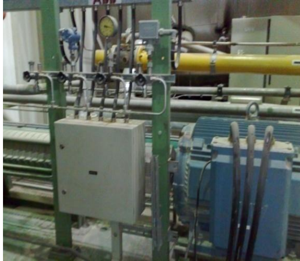
Figure 3.28 At auxiliary boiler room, (GT14)
