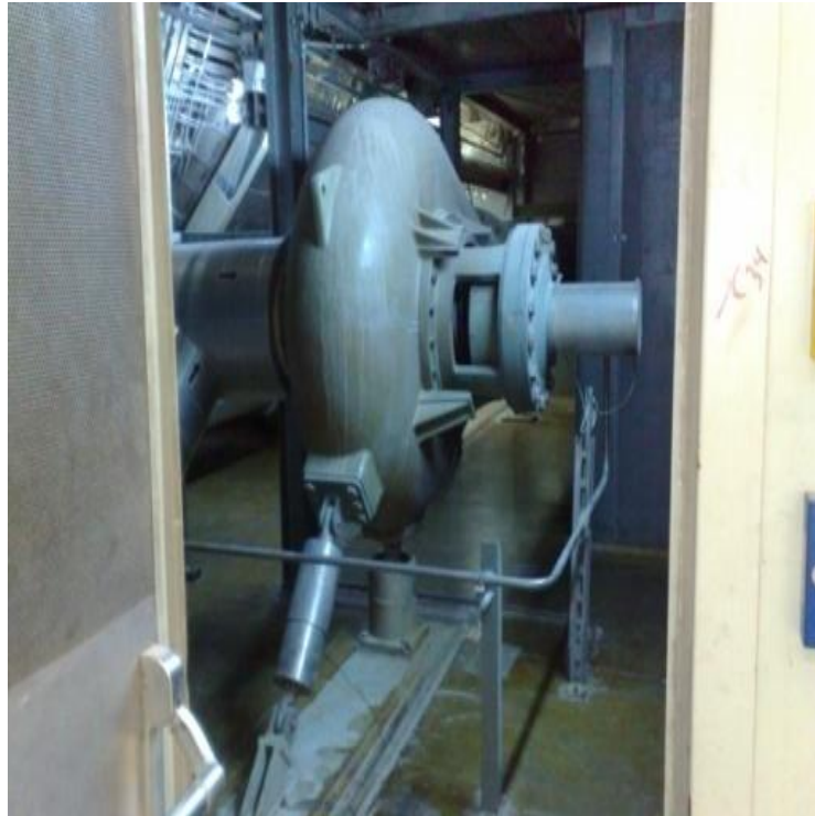
Figure 3.35 At the door auxiliary boiler room 2, (GT14)
