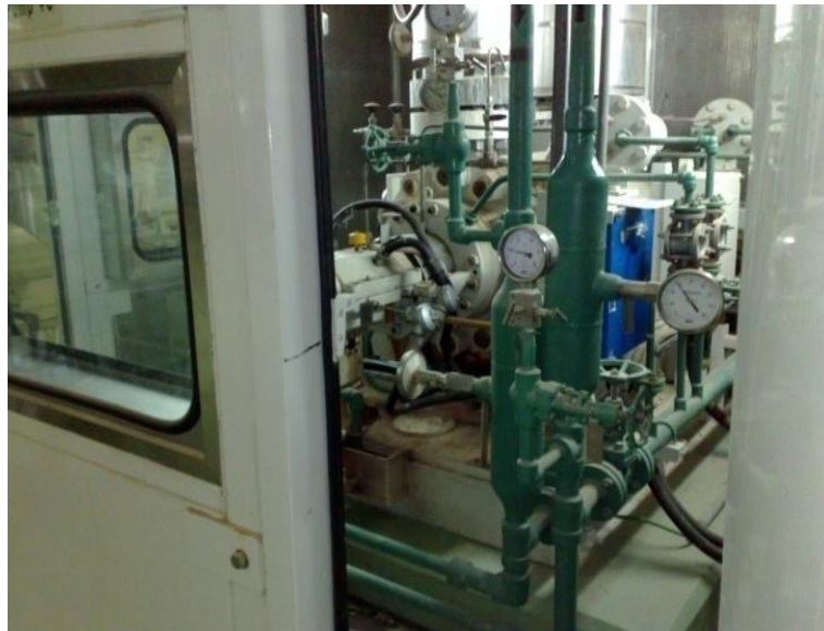
Figure 3.13 At high pressure feed water pump,( STU2)
