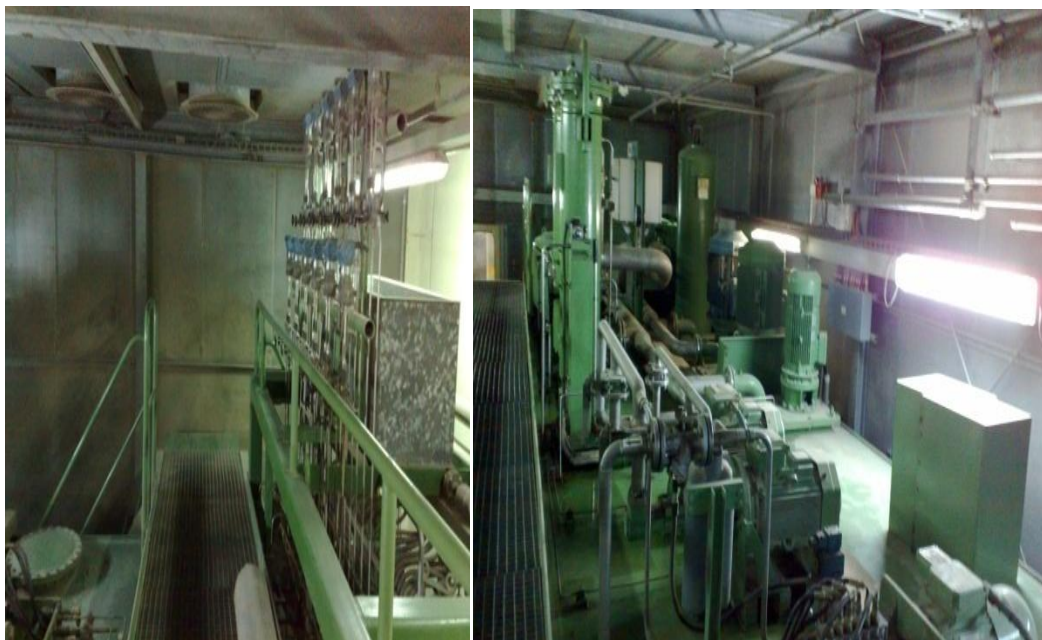
Figure 3.29 Inside (lube oil system) room, (GT14)
