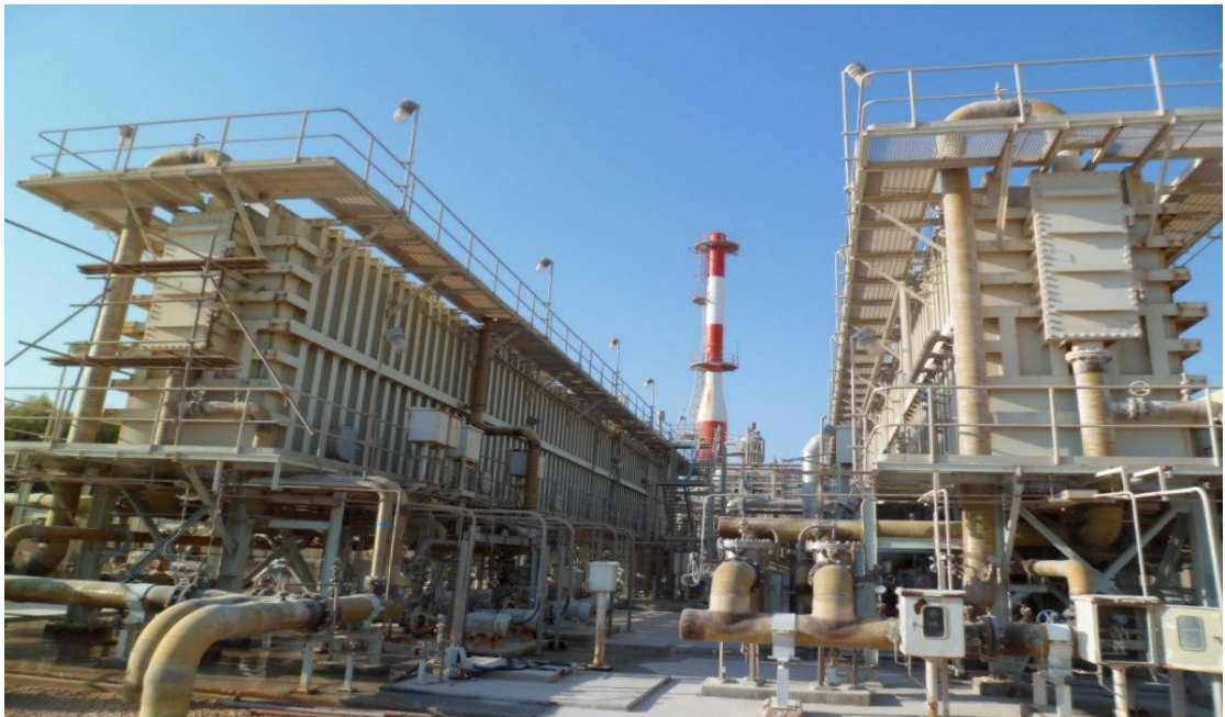
Figure 3.6 MED desalination units (Evaporators) of Zawia power plant
