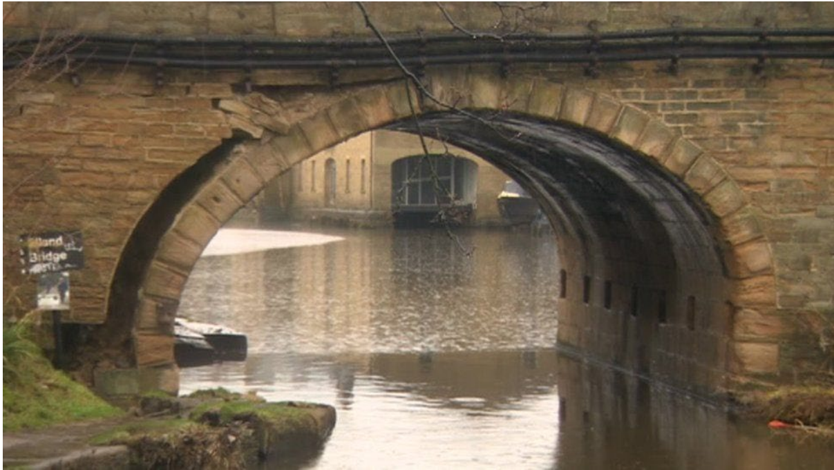
Figure 1-3: Elland Bridge collapsed (BBC News, 2016a).
