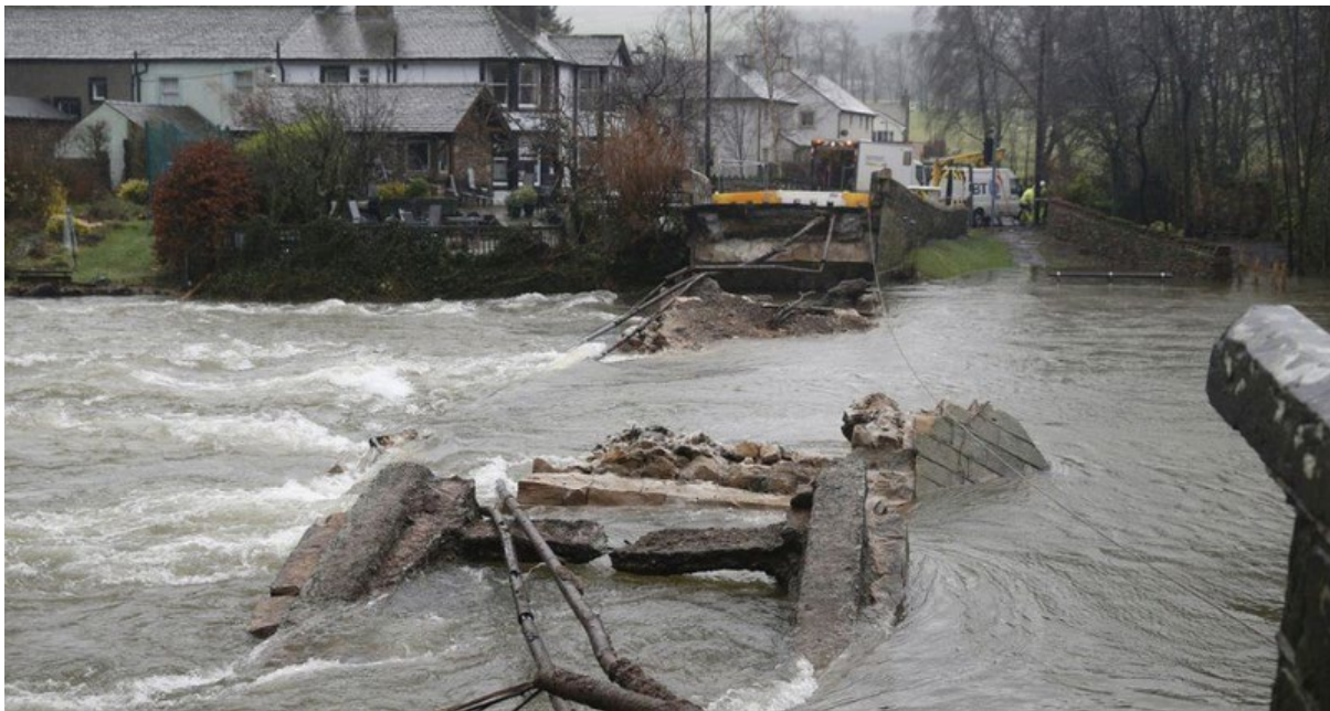
Figure 1-2: Pooley Bridge collapse (BBC News, 2016c).
